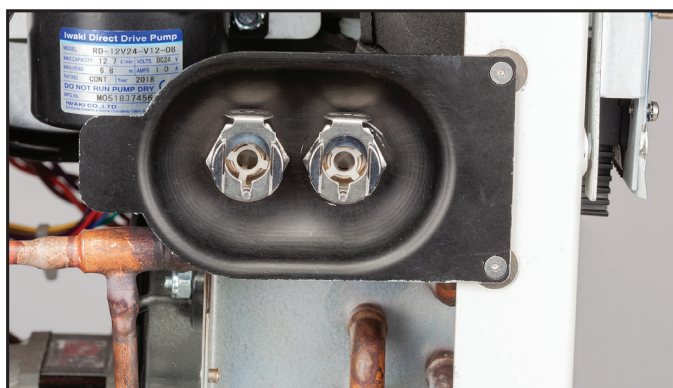
Fig 8-32 Drain Valves at 12 O'clock position in drain cup
